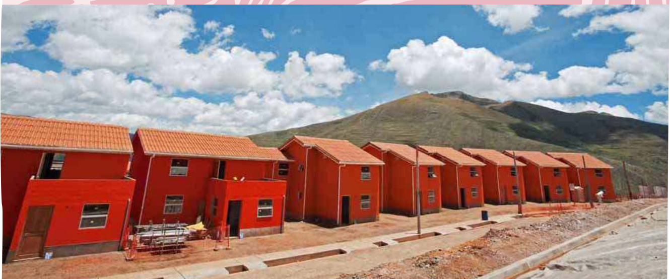
Construction of Nueva Fuerabamba, a community to be inhabited by Fuerabamba families under the resettlement agreement.
