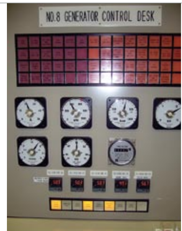
Power generator control desk.
