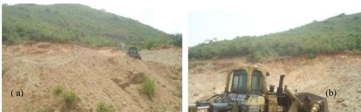
Plate 1 a, b. Threat to Mechisho closure area through excavation.
