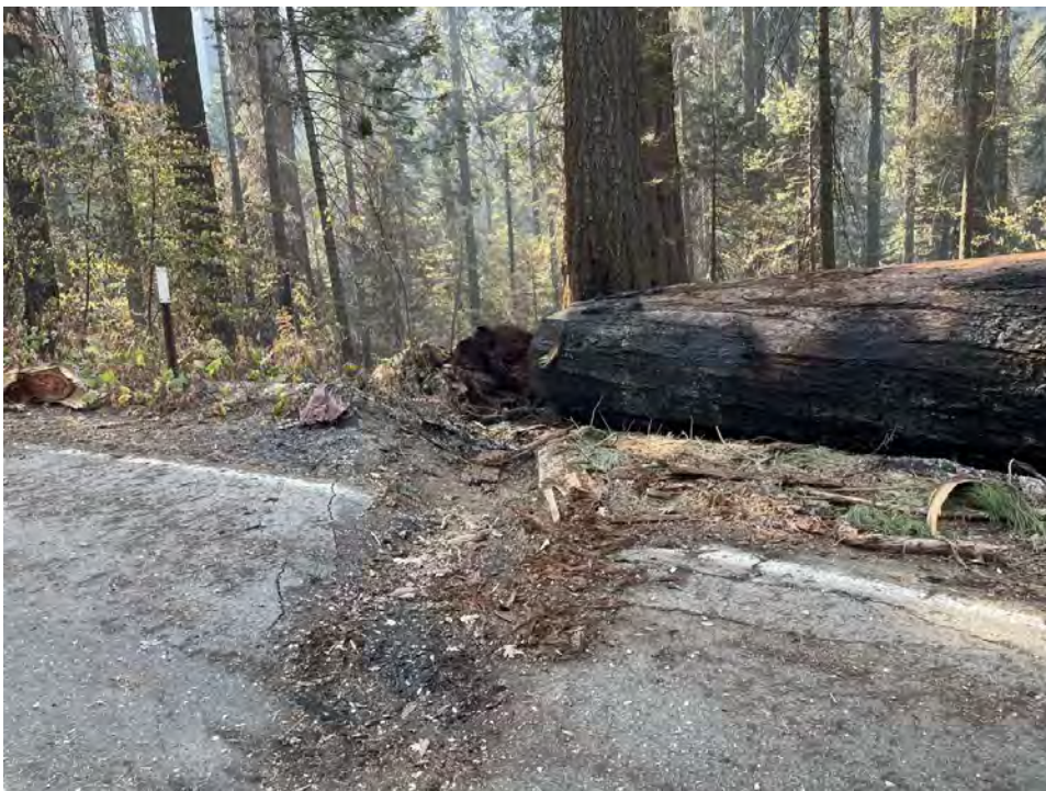
Road damage from Giant Sequoia falling across road near Four Guardsmen Giant Forest
