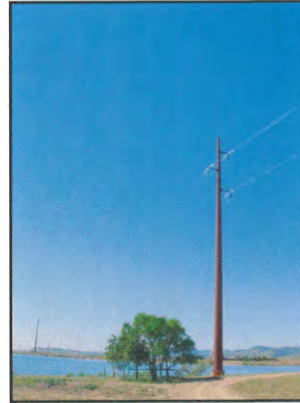
Figure 5: Electric transmission lines crossing over Rocky Flats Lake.
