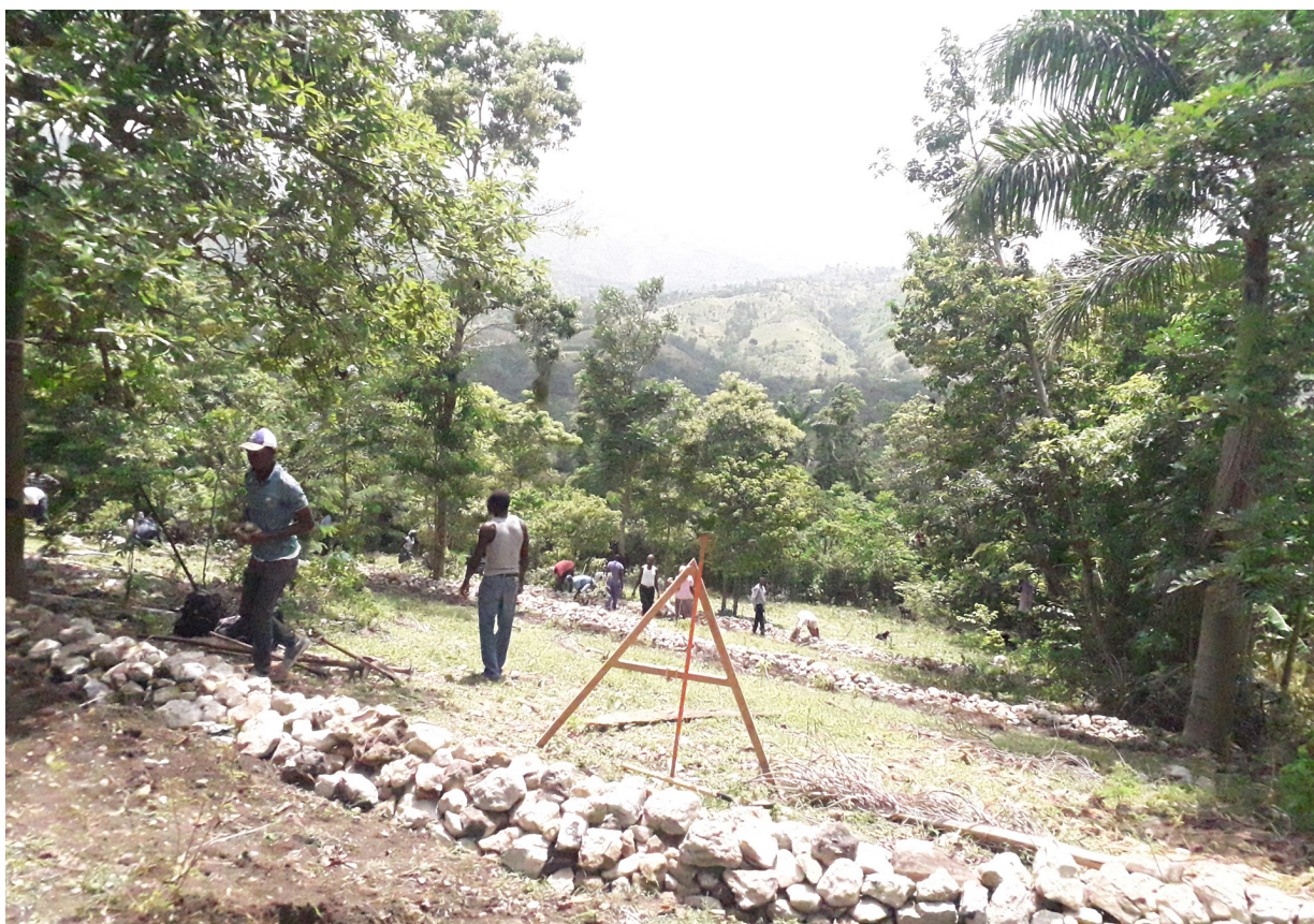
Farmers using A-frame level to build soil conservation contour barriers. Photo by Cantave Jean-Baptiste.
