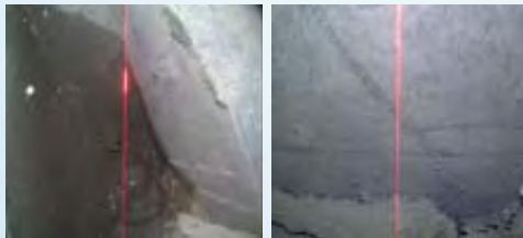
Robot inspecting the lining segments of a tunnel and examples of the images recorded by the cameras.
