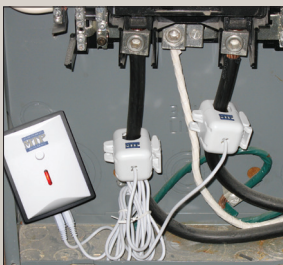
Installation on a standard 200A panel (for total house consumption)
