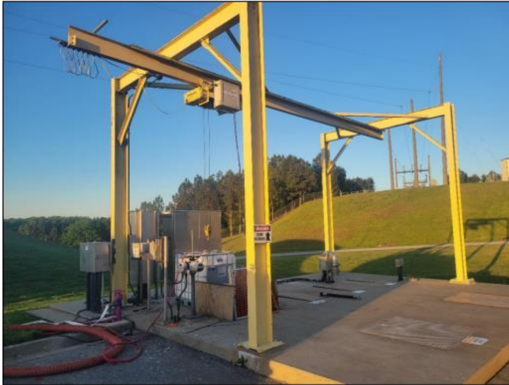
Figure 10: Centrate Pump Station crane
