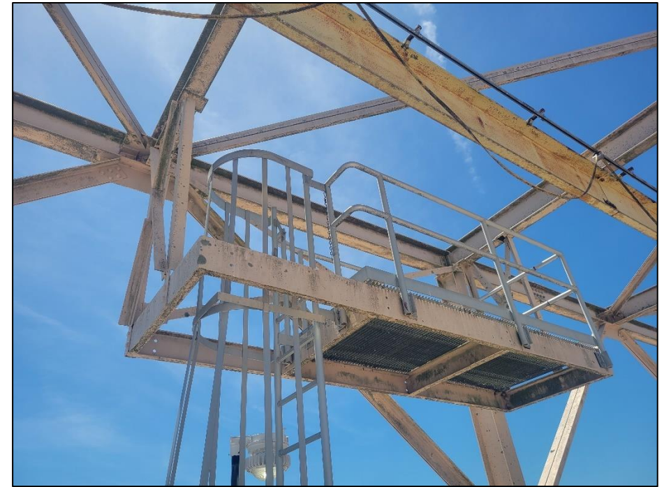
Typical hoist access platform
