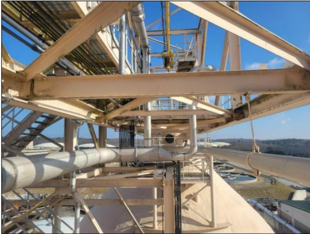
Figure 4: View from intermediate platform of Digester #1 – bottom chords, platforms, truss bridge/walkway looking towards Digester #2. Top chords and hoist beam also pictured at the top of the photo.
