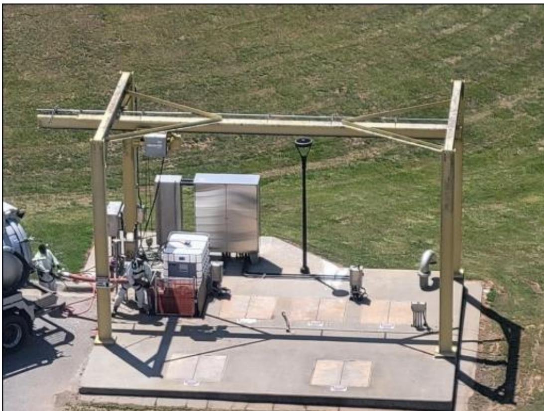
Figure 9: Centrate Pump Station crane
