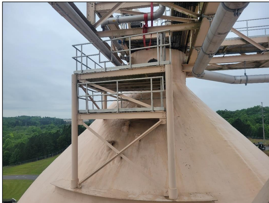
Intermediate platforms typical to Digesters #1 and #2
