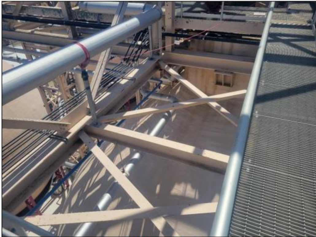
Figure 7: Note many surfaces not easily accessible from platforms. Also note, some pipe support hangers are coated, and some are galvanized. Coated hangers shall be recoated.
