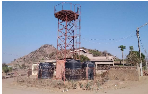
HCB's water supply system in the Unidade neighborhood
