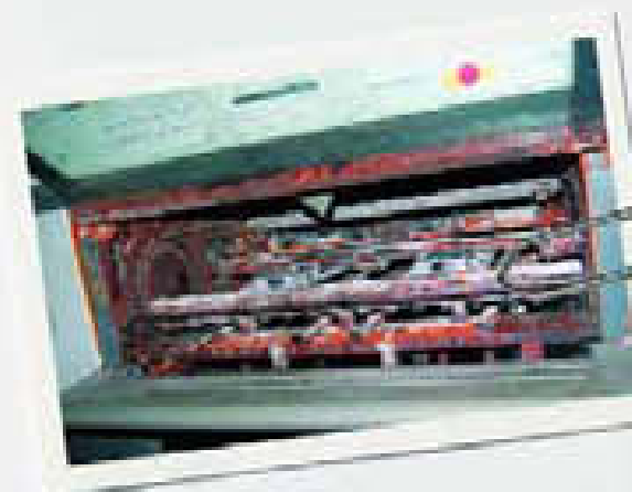
In the shortest time possible, the flood corroded the electronics in all of the equipment, for example on the POLAR cutter (photo on top), and the printing press. (photo below)
