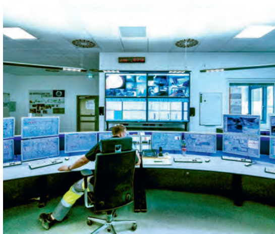
Plant control is now completely digital, as shown here at the Lengfurt plant, circa 2020.
