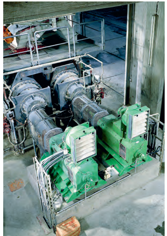
High-pressure grinding rolls at the Schelklingen cement plant, 2000
