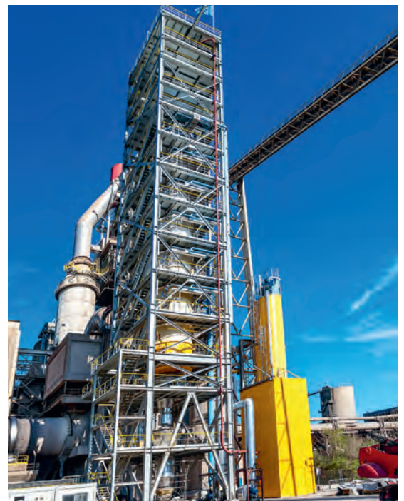
Demonstration calciner at the Lixhe plant in Belgium for the capture of high-purity CO 2 , 2019
