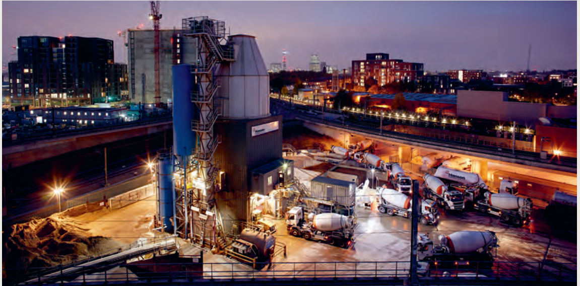
Ready-mixed concrete plant for construction sites at Kings Cross in London, 26/10/2015
