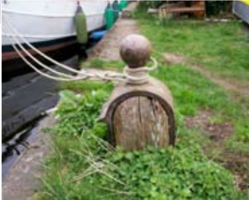
Mooring Bollard, Shannon Harbour. © (Helen Kelly)
