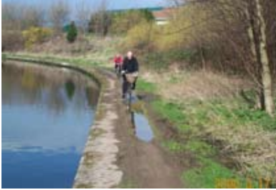
Narrow rutted towpath at Beeston, west of Nottingham city centre, prior to improvement © (Roger Butler)
