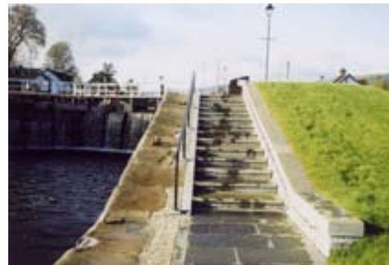
New steps at Fort Augustus lock flight, incorporating high quality stone work, paving and reprofiled grass banks. © Roger Butler
