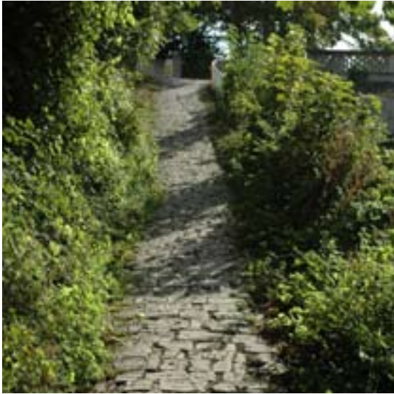
Built heritage includes original towpath surfacings, such as this stone paved ramp in Bath. The restoration work ensured such features were retained and conserved. © Roger Butler
