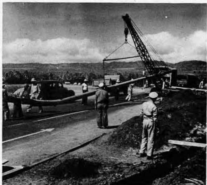
MOVING ALONG a busy highway, a crane is shown maneuvering a heavy long piece of pipe. Not one flaw has been reported in the entire 11 miles of line.
