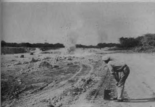
BLASTING FOR CORAL at one of the island's numerous airfields. 16th Seabees helped enlarge, repair and maintain important air strips on this teeming island.
