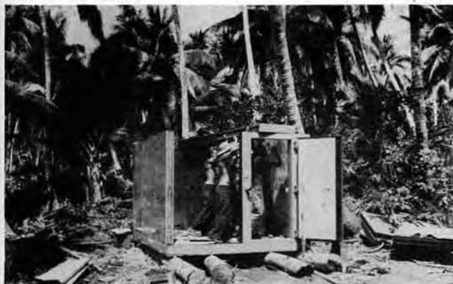
16TH SEABEES SETTING up first reefer on Island "X." Cold drinking water was a luxury and like most everything else at the island outpost had to be rationed. Canteens were usually filled under the friendly cover of darkness.
