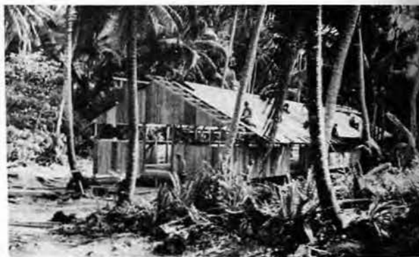
IN THE MIDDLE of a thick jungle setting, 16th Seabees Nukufetau rush construction of the first mess hall. A build of this type is usually completed in one day.
