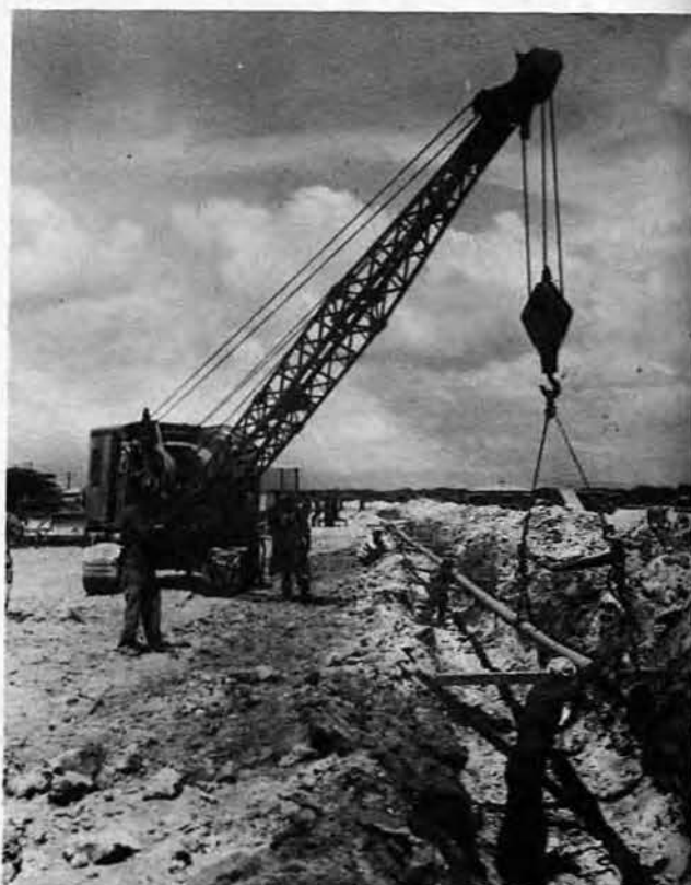
A GENERAL IDEA of the terrain covered during this project is shown in picture above. Majority of the line was laid in road shoulders where jack hammer operators had to chisel through coral rock.
