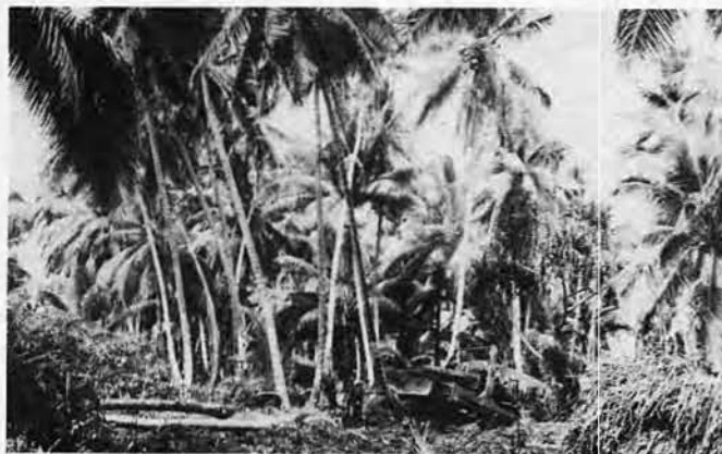
TIMBER! A roaring, power-packed bulldozer rams another coconut tree to make way for the planned air strip. During the early stages of the work on island "X" 16th Seabees worked feverishly from 12-18 hours daily.
