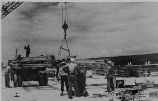
THE FIRST MAJOR construction assignment tackled by the Fighting-Building Sixteenth Seabees was the erection of warehouses, repair shops and utilities at an island base. This picture was made on the 15th of October, 1942.
