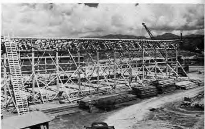
STILL ANOTHER VIEW. Sixteenth Seabees hit the ball on this important project, turning over first warehouses to Naval Supply one month ahead of schedule. For more pictures of Gulch project see following pages.
