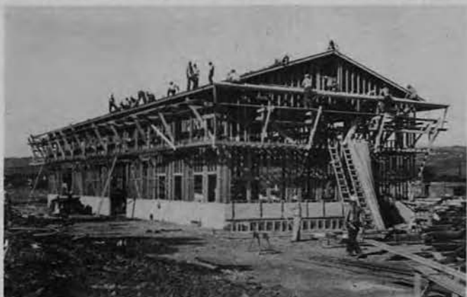
HALF COMPLETED when this picture was made, busy Seabees are shown finishing the roof while others swarm around the sides ready to start work on the bulkheads. This area was later used as battalion operating base.
