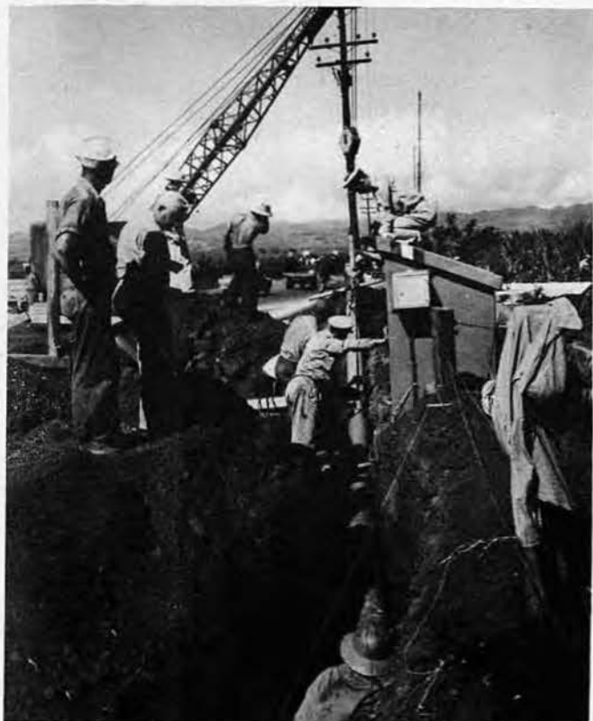
NOT TO BE OVERLOOKED as a vitally important war-time project was the laying of the gas pipeline by Sixteenth Seabees. This major job was undertaken in April 1943.
