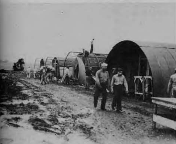
ON MARCH 10, the battalion moved from tent city to a Quonset hut camp constructed nearby. Some few months later, when the camp had been developed into one of the finest of its kind the battalion was moved to a new area.
