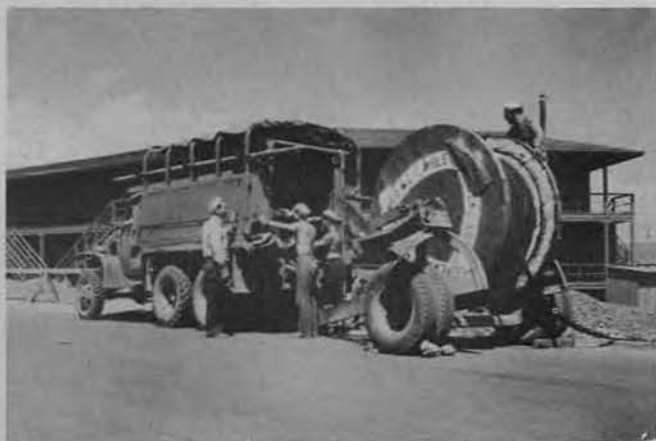
ANOTHER VIEW of 16th Seabee electricians at work on the cable project. These same men were later called upon to install and erect radio towers, huge switchboards and power plants.
