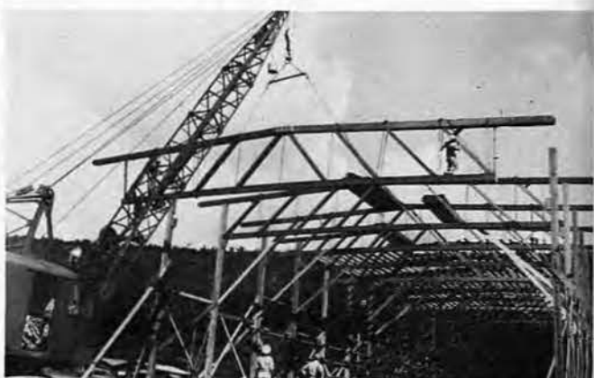
HERE A HUGE CRANE is shown setting one of the trusses into place on the first warehouse.
