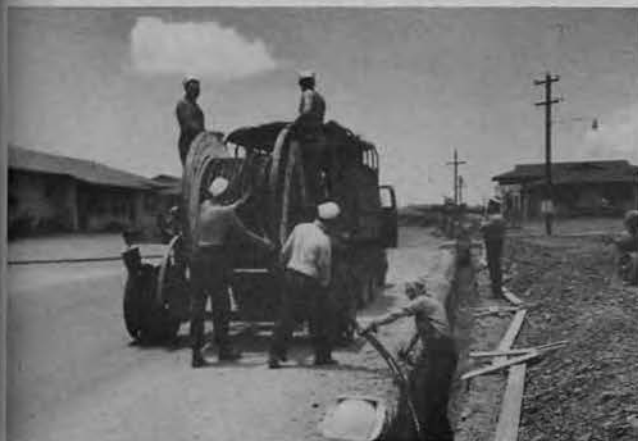
CABLE LAYING PROJECTS were numerous during the early days overseas. 16th Seabees are shown above laying heavy cable in area near Pearl Harbor.
