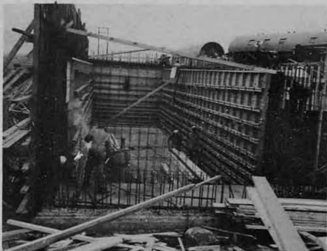
ABOVE PICTURE SHOWS side view of 6000-man septic tank constructed by 16th Seabees at new island Quonset camp. This was the first major project undertaken following the battalion's return from down below.
