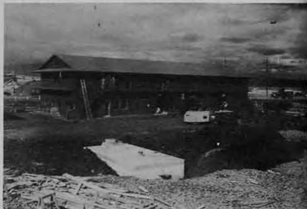
PICTURE ABOVE SHOWS the first completed warehouse. 60 x 160 feet in size, the battalion later completed a similar building and also added smaller buildings including huge repair shop.
