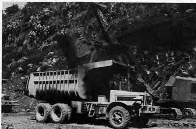
FOLLOWING BLASTS like the one shown above, huge shovels and trucks were employed to clear the rock later to be used for the road bed. Truck shown in picture is 25-yard dump—the very largest of its kind used on the island.
