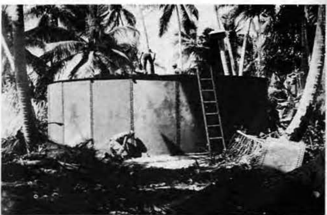
THE FIRST OF SEVERAL huge fuel storage tanks nears completion at Island "X."
