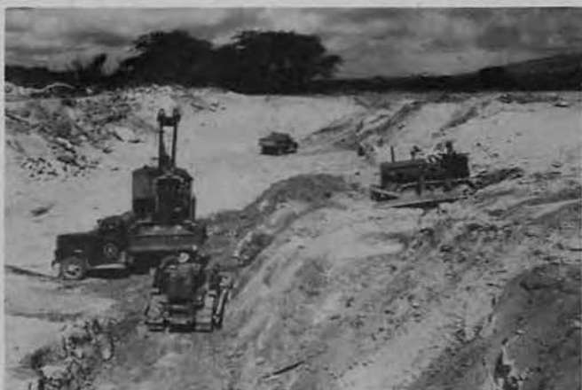
HUGE CORAL PITS similar to the one shown above were worked day and night by battalion powdermen and heavy equipment operators.
