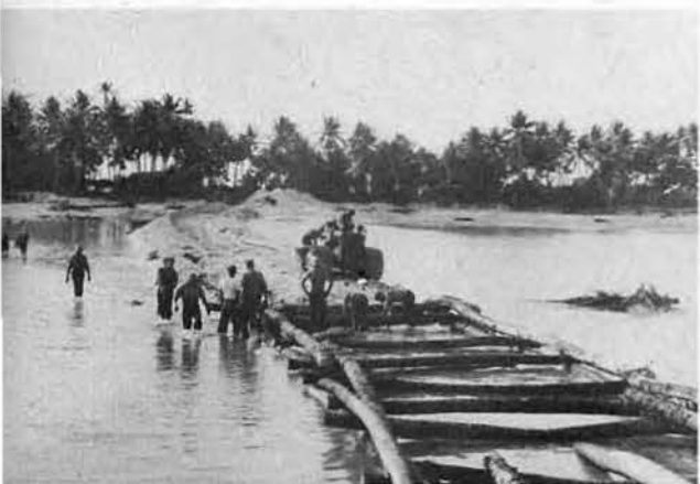
SOME WEEKS LATER huge rocks were blasted away and holes filled as Seabees prepared to build coral roadway from the shore to reef.
