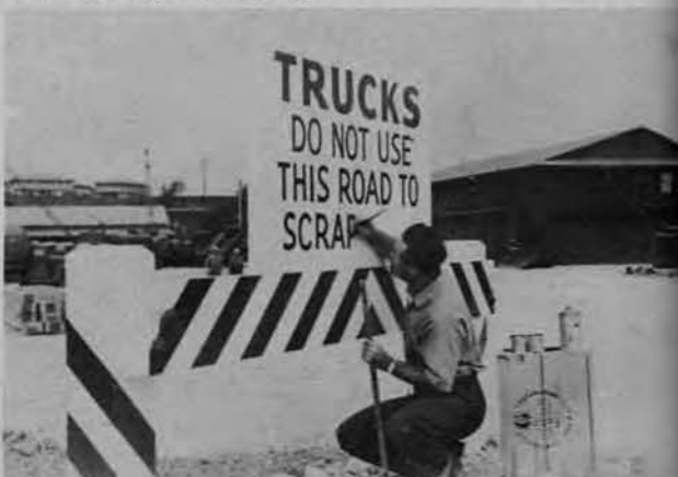
JACK WATSON, battalion painter, is shown adding the finishing touches to the completed project. Complete water and sewage system, plus all electrical installations were designed and completed by 16th Seabees.
