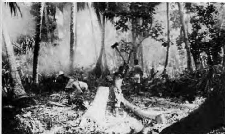
NATIVE WORKERS shown above are helping 16th Seabees clear camp area. Strong, tireless men, their assistance was invaluable during the early stages of the operation. Paid on the British wage scale, they received two shillings or 33 cents per day.
