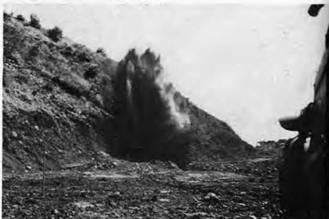
INCLUDED IN THE PROJECT was the construction of a one and one-half mile, three lane, paved roadway. Dynamite blasts similar to the one shown above helped to clear the way for road graders.
