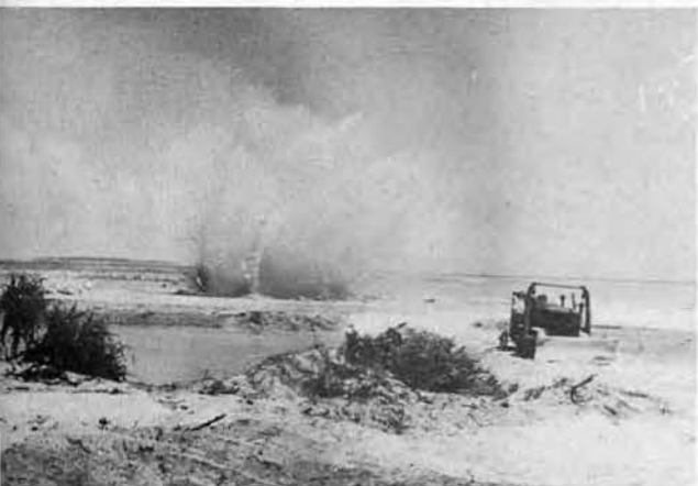
FOLLOWING UP the working crews, bulldozer operators filled the "cribs" with coral rock. Roadway was three-quarters finished when this picture was snapped.
