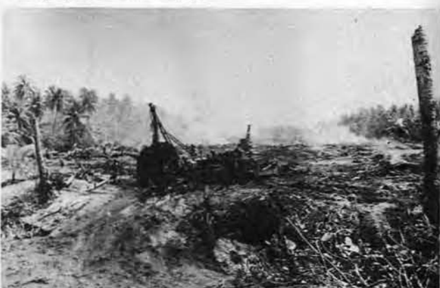
BULLDOZERS, CRANES and trucks clear debris as numerous fires are set to burn out underbrush and coconut fronds. Men worked long 12-hour shifts under a blazing sun while equipment rested only when taking on fuel.
