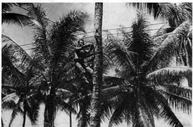
ELECTRICIAN MATE Frannie Oliver climbs a coconut tree shooting for trouble on the island's communication system. Heavy winds and numerous tropical storms kept the linemen busy.
