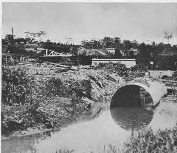
One of many drainage problems encountered.
