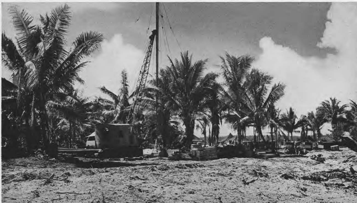
Erection of antenna tower on edge of dense cocoanut grove at Bear Point.
