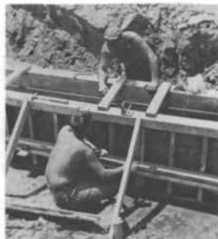
Setting forms at the Port Facilities in Da Nang are (L-R) J. E. Womak, and C. Hoken. The large port facilities heads the list of important projects undertaken by USN MCB-EIGHT.
