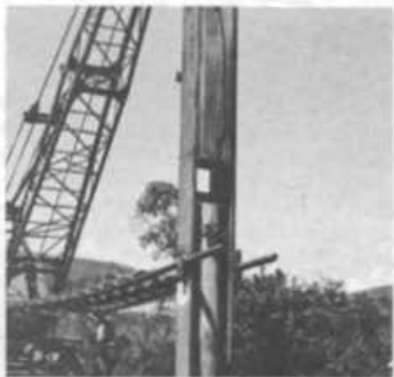
Close-up showing the leads of the pile driver, and the catwalk extending from the base of the crane's boom out to the pile driver leads. The rig can be assembled or disassembled in about 10 minutes.
