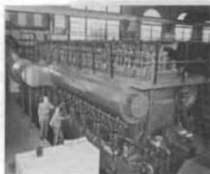
8725 bhp, 6250 kw Nordberg Series 21 engine installed at Carthage, Mo., municipal plant.
