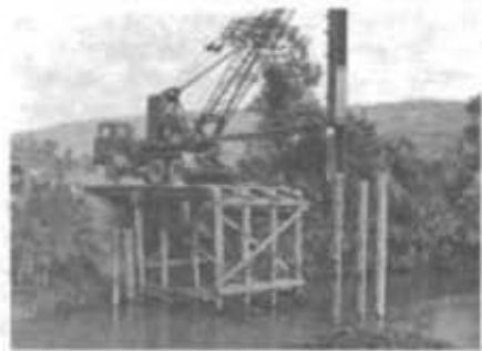
The 'home made' pile driver set up to begin operation on the Da Nhim River in Viet Nam
