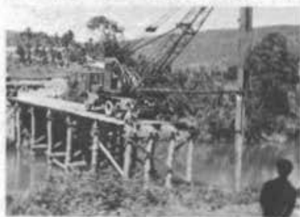
Part of the 36 piles are shown as the bridge rapidly approaches completion. Another example of the Seabee's ability to improvise.
