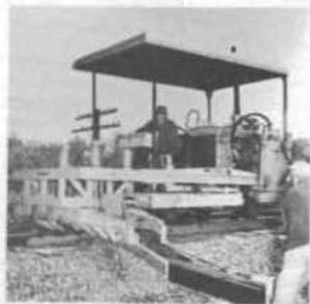
Scarifier-Inserter on test on the Northwestern track outside of Des Plaines, Illinois.
