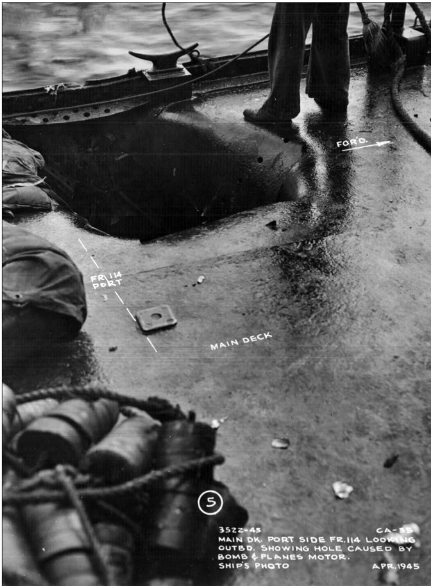
Figure 1-1. Hole in main deck caused by Japanese bomb at Frame 114 port side.
