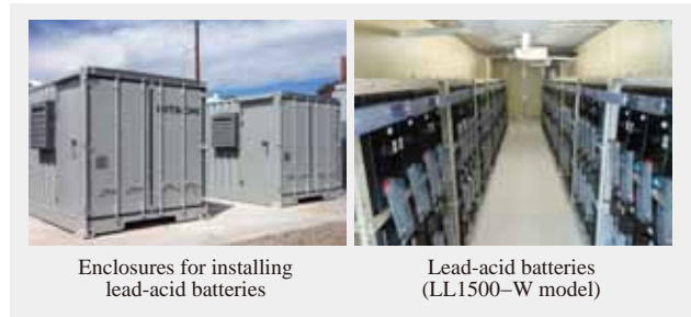
Fig. 7—Lead-acid Battery System Installed in Los Alamos County, New Mexico, USA. The lead-acid battery system installed in a Japan-U.S. Smart Grid Collaborative Demonstration Project in Los Alamos County, New Mexico.
