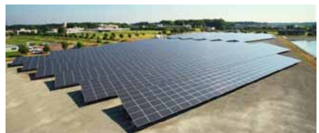
Fig. 1—Large Photovoltaic Generation System (Ibaraki Prefectural Public Enterprise Bureau).
