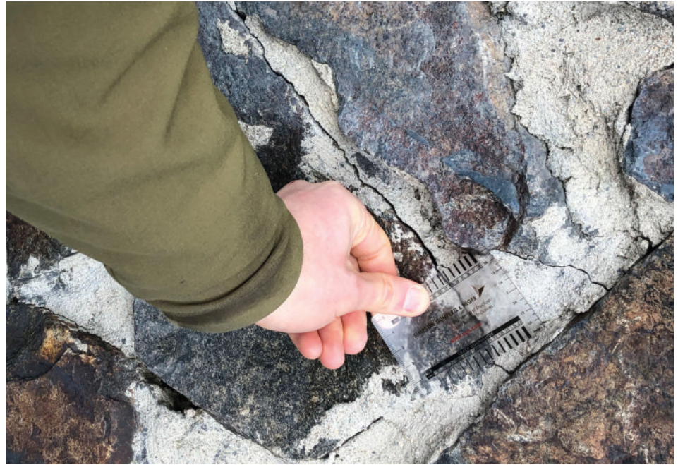
Crack width measurement at stone masonry retaining wall
