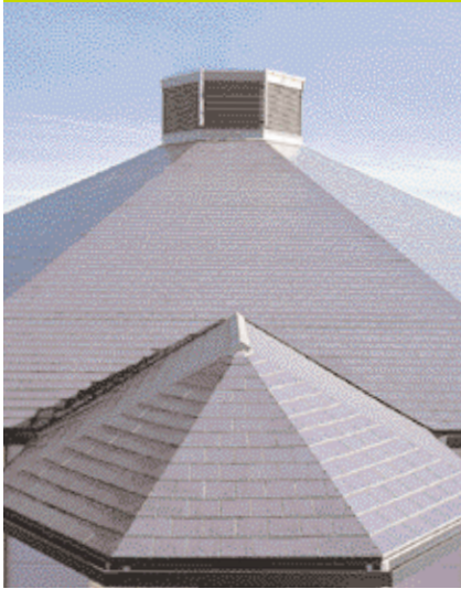
UNITED KINGDOM | Roofing | Cambrian Slate roofing tiles on the University of Bournemouth library
