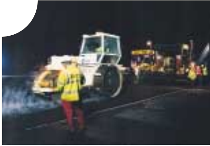
United Kingdom – Laying of asphalt mix on a runway at London's Gatwick Airport
