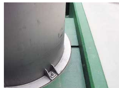
Leakage monitoring well at base of solvent tank
