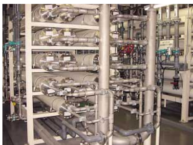
Wastewater recycling facilities at Mie plant
