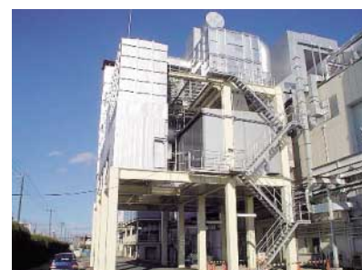
Waste gas processing equipment installed at the Gunma plant
