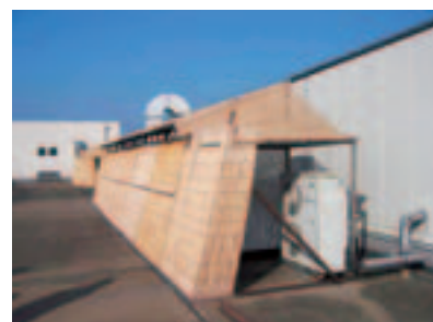
Measure to assure the effectiveness of the air-conditioning system by shielding the outdoor components from direct sunlight (sunshade)
