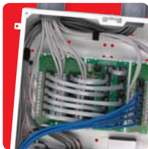
HOME WIRING & NETWORKING
