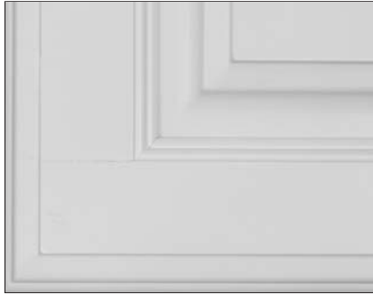
Example of door front joint separation
