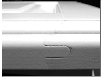
Example of door end joint separation
