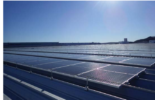
Saitama Factory's assembly plant (2.0 MW)
