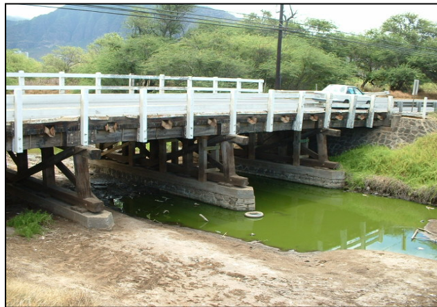
Mākaha bridge drains mauka water into the near shore area.
