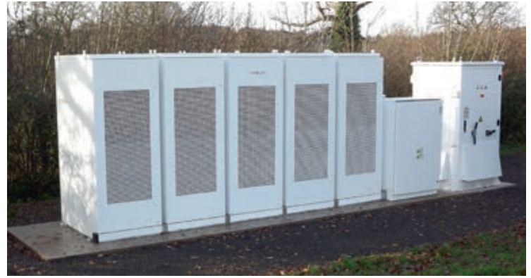
Some of the first Tesla Powerpack batteries in the UK have been installed in Somerset.
