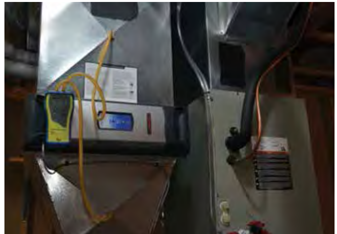
Install cabinet-style air filters horizontally wherever possible to improve serviceability and remove the need for turning vanes in the return air boot. Installing a low initial \Delta P filter means less energy is required to move air through the system.
