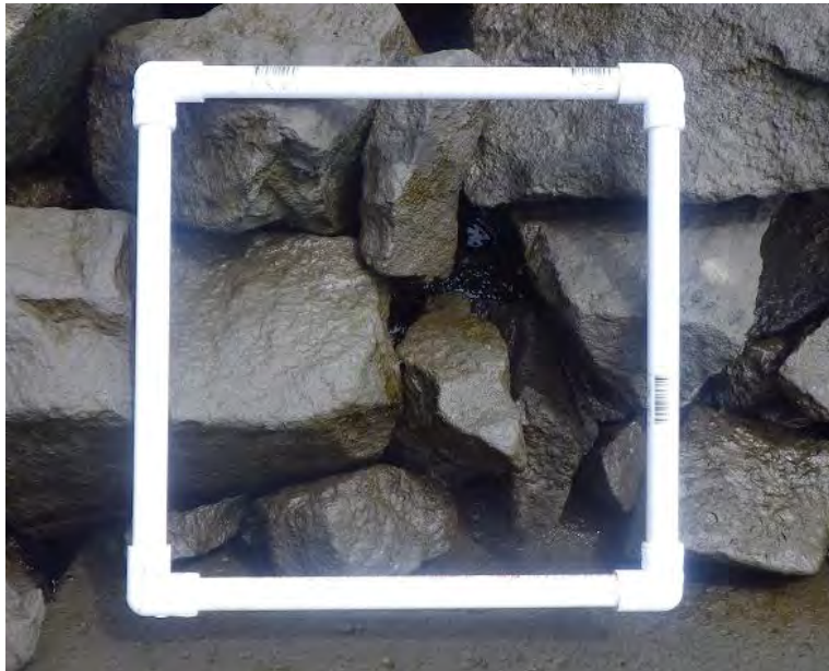
Figure 11: A quadrat (0.25 m x 0.25 m) placed in the intertidal zone of the riprap shoreline at Harlem River Park. As with other shorelines around Manhattan, the intertidal zone was covered in fine deposited sediment, without identifiable animals or algae on the upper surfaces of rocks.
