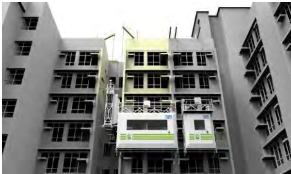
Figure 10. The multifunctional façade-processing robot showcasing the painting function on the façade of public housing buildings in Hong Kong (image: R. Hu)
