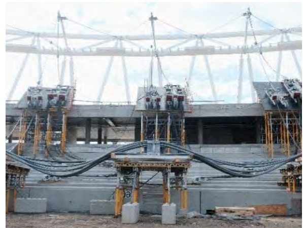
Figure 6 The cables before the strain
