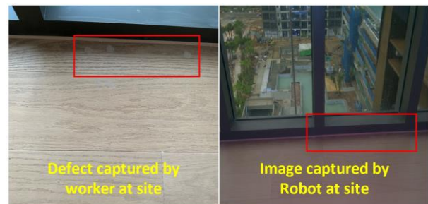
Figure 12. Some defects not observed from far distance with bad light conditions
