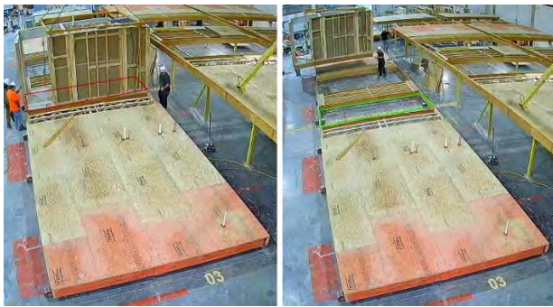
Figure 10. Installation of bath pod, as detected in the pre-planned location, on the modular unit
