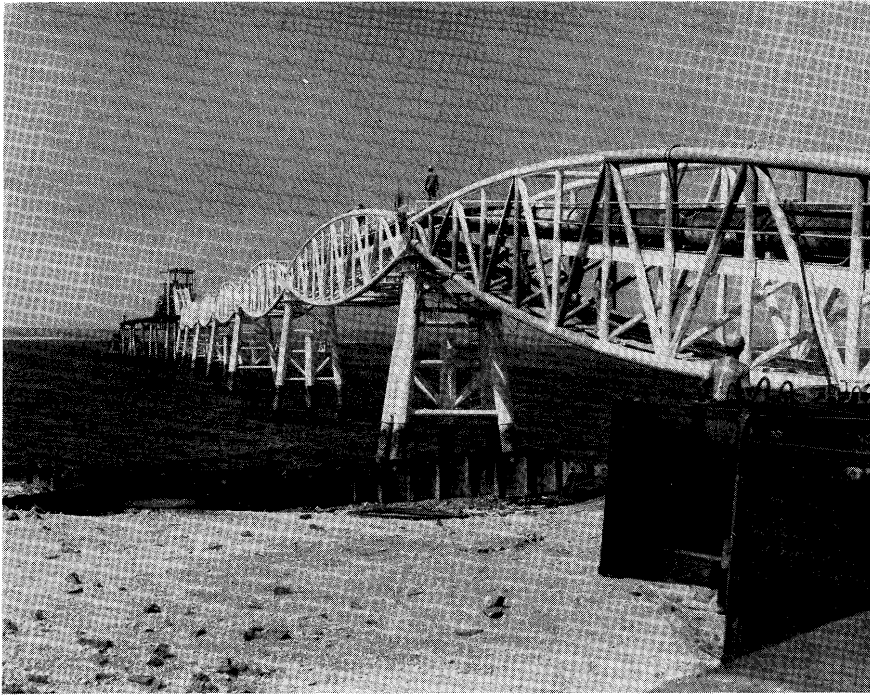
6. Conveyor trestle supports temporary pipeline carrying a mixture of sand and water.
