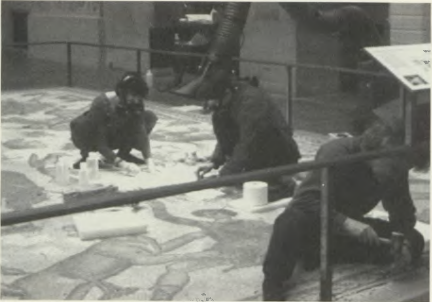
4. Conservation team in 2002 chiseling out cement fills and removing a polyurethane coating.
