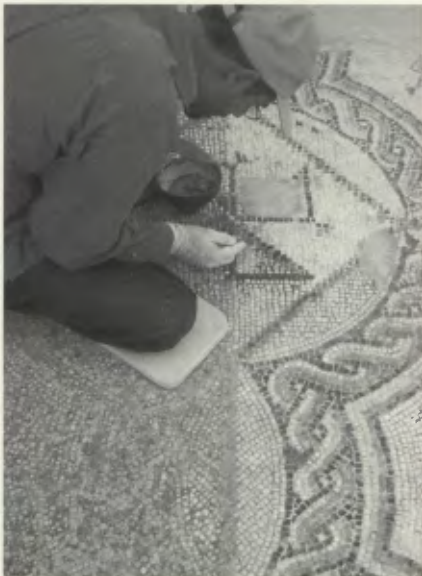
4. Peristyle of the Maison de Neptune at Thurburbo Maius, trainee carrying out mortar filling of interstices after cleaning.
