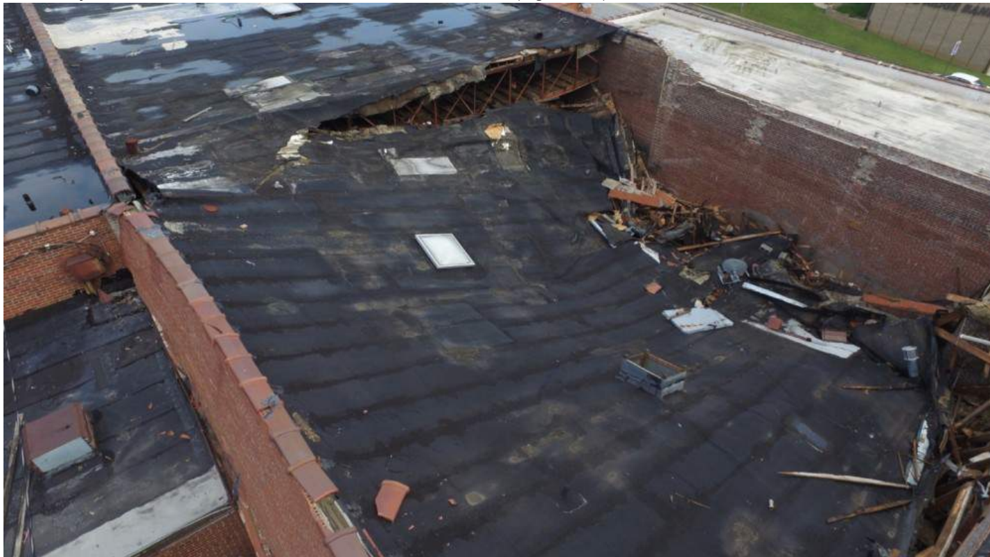
Case Study 1: Roof Failure in Walhalla, South Carolina, on October 8, 2017 (Figures 3-4)
