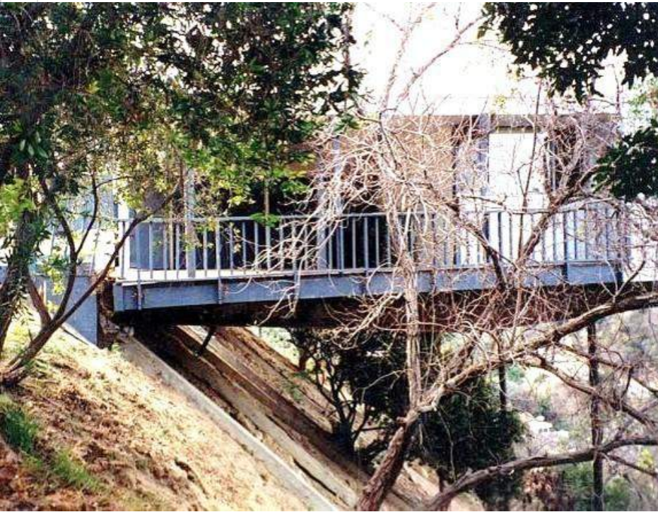
Figure 3. Hillside building pulled away from uphill foundation in the 1994 Northridge, California Earthquake (Credit: City of Los Angeles Department of Building and Safety). Red arrow shows location where floor framing has pulled six to eight inches away from the uphill foundation.
