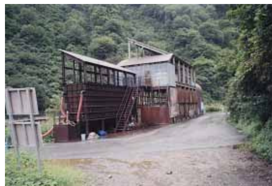
Photo 4 Muddy Water Treatment System (Processing Capacity of 200 m 3 /h)
