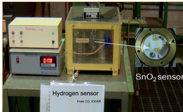
Fig. 1 Photograph showing the installation of SnO 2 sensor at the thermal conductivity detector outlet in the secondary sodium circuit (west) of FBTR
