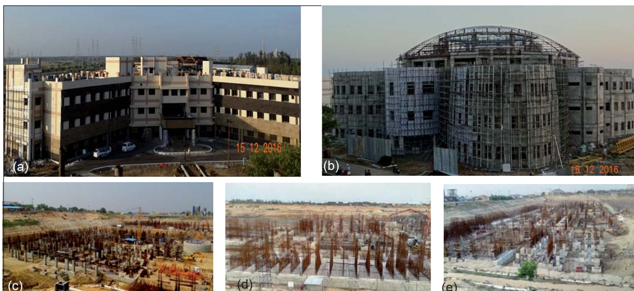
Fig. 1 (a) Waste management plant, (b) fuel fabrication plant, (c) core sub assembly plant, (d) administrative building and (e) training centre
