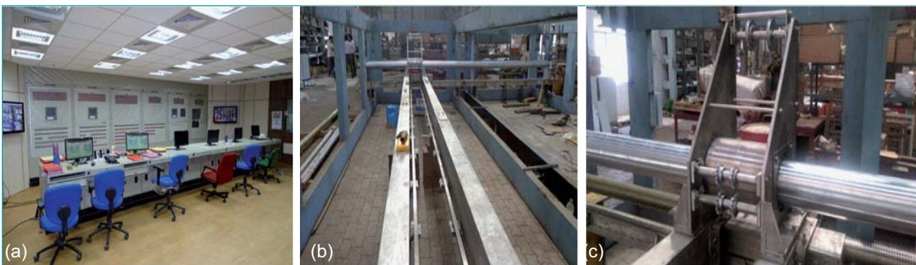
Fig. 2 (a) View of main control room and (b) and (c) special in-cell crane for dissolver cell of DFRP
