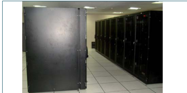
Fig. 1 Server cabinet with rear door heat exchangers
