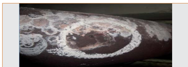
Fig. 1 The bend portion of the feed water line downstream to steam generator
