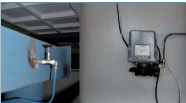
Fig. 2 Pressure tapping and pressure switch
