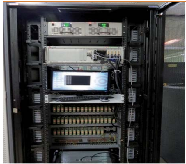
Fig. 2 Commissioned system process disturbance analyzer
