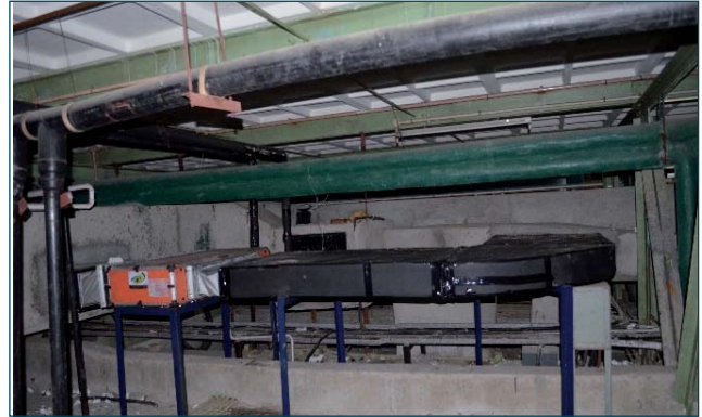
Fig. 1 Fan coil unit with ducting/piping
