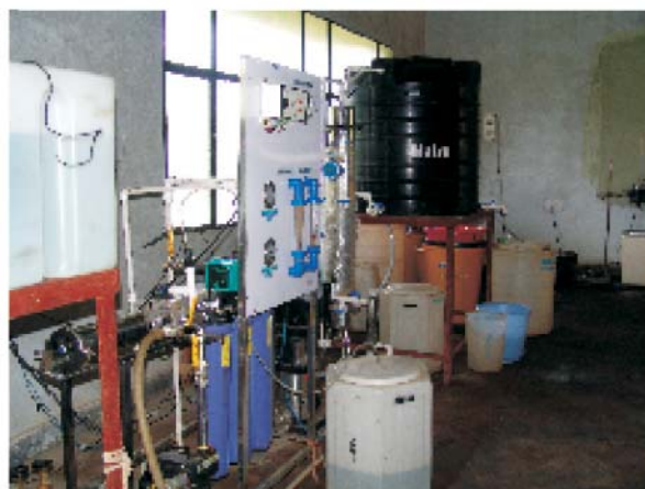
Water purification system
