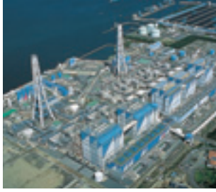
Boilers for power plants
