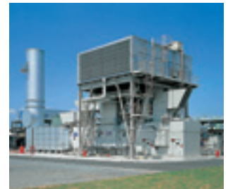
Gas turbine power plants
