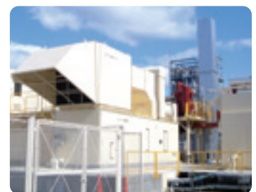
Gas turbine co-generation facility
