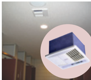
Ceiling-mounted deodorizing systems
