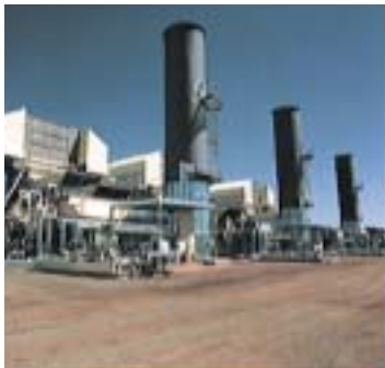
Gas turbine cogeneration systems
