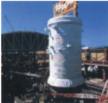
Reactor pressure vessels
