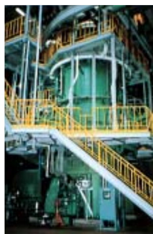
Vertical coal pulverizer for coal-fired thermal power station
