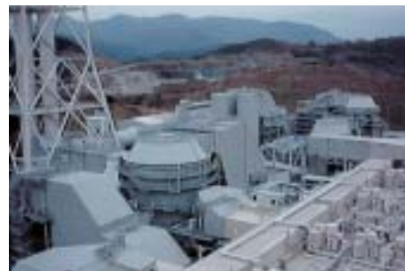
Flue gas DeSO x system for 700-MW power plant
