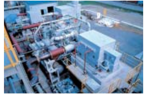
Large-scale turbo compressor for liquid nitrogen production plant
