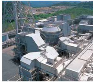
Air pollution prevention systems
