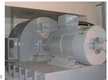
Flywheel power storage system
