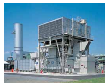
LM6000 gas turbine power generation facility
