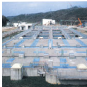
Sewage treatment systems
