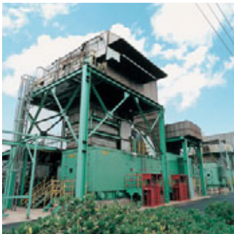
Gas turbine cogeneration systems
