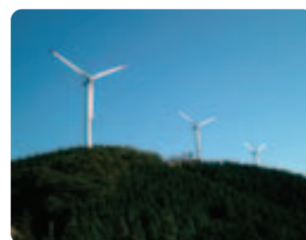
Wind turbine generators for Muregaoka Wind Farm
