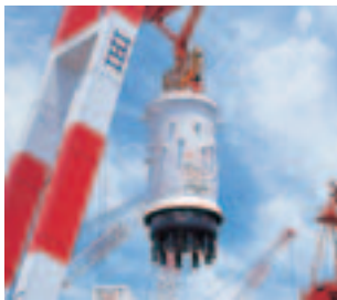
Reactor pressure vessel
