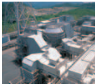
Air pollution prevention systems
