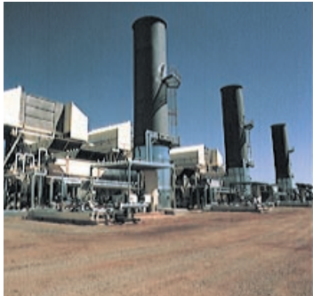
Gas turbine cogeneration systems
