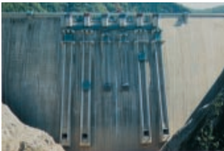
Gates for domestic multipurpose dam
