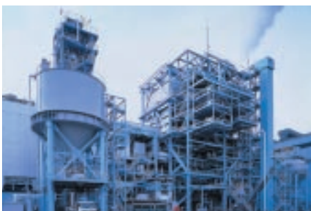
Boiler for 145-MW-class IPP power plant
