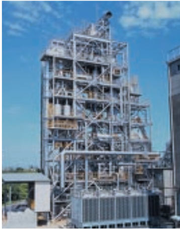
Demonstration plant for RDF-fired external circulating fluidized-bed boiler
