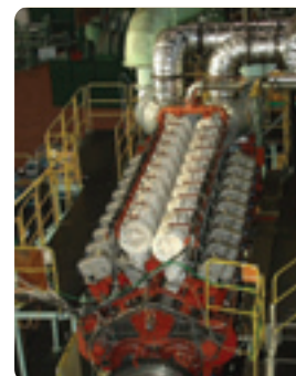
Large gas engine 18V28AG
