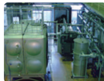
Heat recovering system
