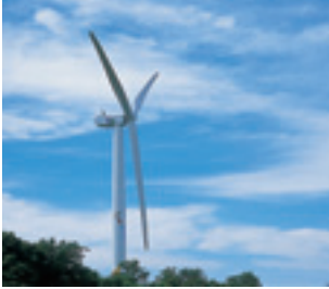
Wind power generation systems
