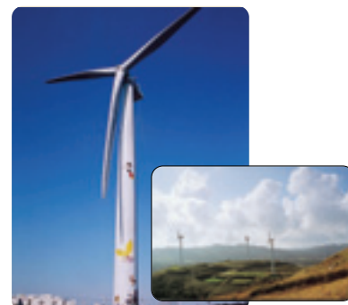
Wind-turbine generators for Minami Osumi Wind Farm (right) and Wakasu Seaside Park (left)
