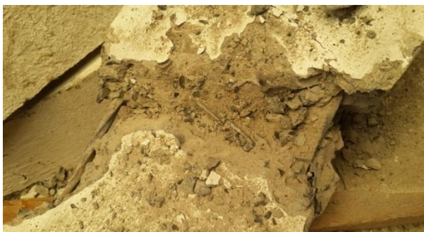
Figure 16: Snapped shear reinforcement for steel 1x6 beam
