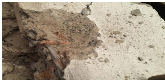
Figure 8: Unbroken shear reinforcement for L.B.1x6 beam
