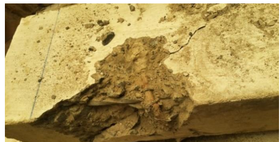
Fig.10: Unbroken shear reinforcement for L.B.1x8 beam
