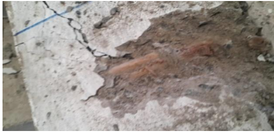
Figure 12: Unbroken shear reinforcement for L.B.2x10 beam
