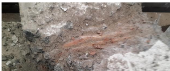
Figure 14: Unbroken shear reinforcement for L.B.2x13 beam
