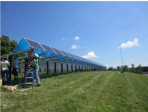
Wright-Hennepin Community Solar, MN Source: Clean Energy Collective
