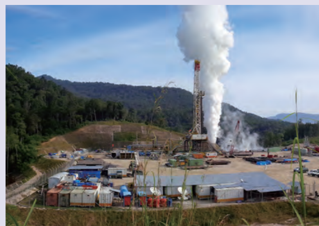
Fumarolic testing for the Sarulla Geothermal Power Generation Project
