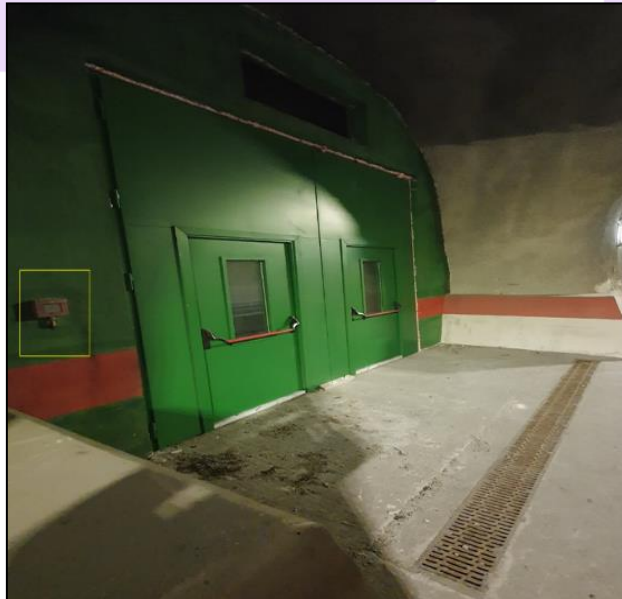
Figure 4. Service hose for evacuation of endangered persons
