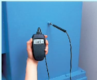
Measuring airflow rate inside duct
