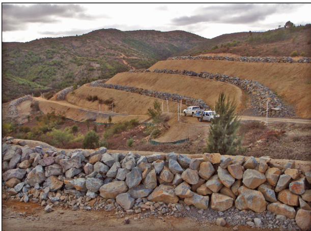
Fig. 3. Rock reef habitats being constructed in the prospective inundation zone of the enlarged reservoir
